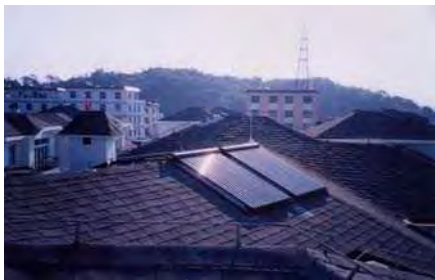
Figure 10: Dual collectors on roof
