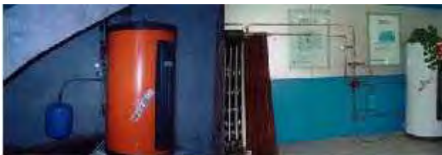
Figure 20: Solar Water Storage tank with plumbing
