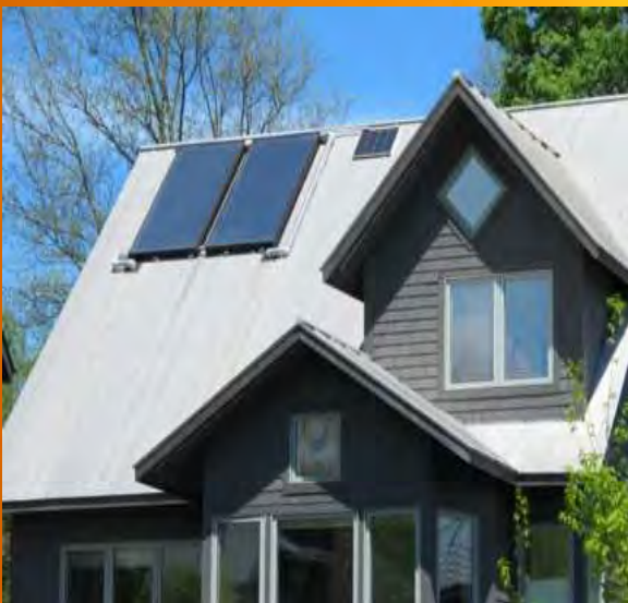
Small PV panel for pump beside solar water thermal panels.
