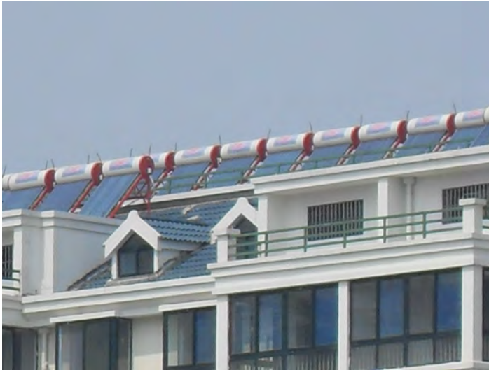
Figure 9: Multiple integrated solar systems on roof of apartment building
